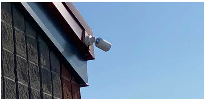
PCI Datacenter security
